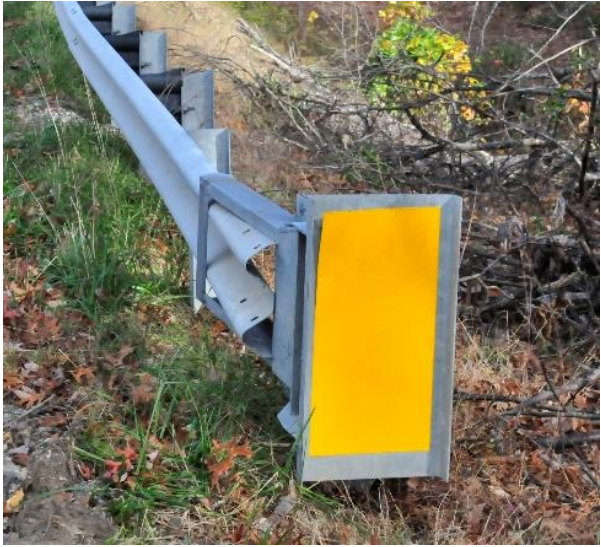
Improper Seating of Rail into Head
