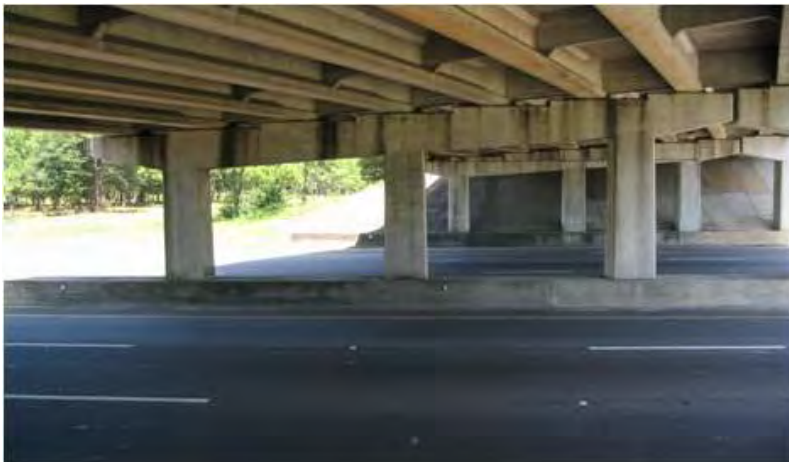
Photo 9: Staining on sides of pier caps
