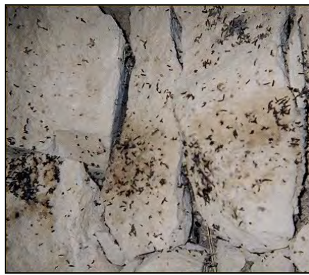
Photo 6: Bat Guano on Riprap
