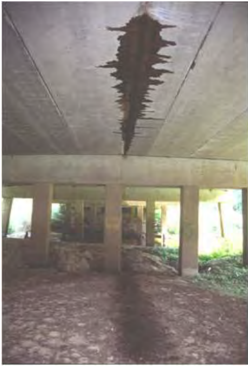
Photo 7: Staining along longitudinal joint. Guano deposits on the ground.
