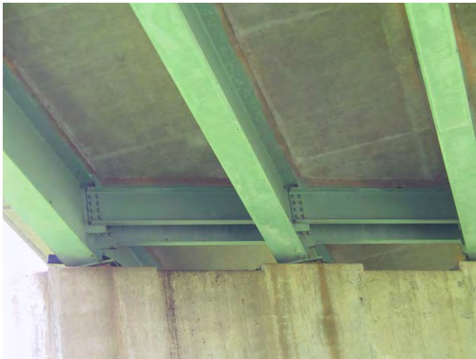
Photo 10: Guano staining on side of pier
