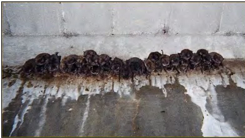
Photo 11: Bats roosting & associated staining
