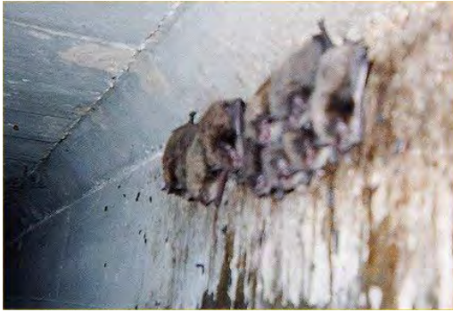
Photo 1: Bats hanging from cracks along support beams
