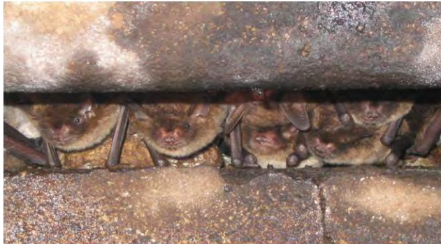
Photo 2: Visible bats within an expansion joint
