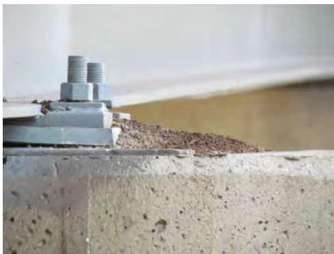
Photo 5: Guano deposit on pier, obscuring structural features.
